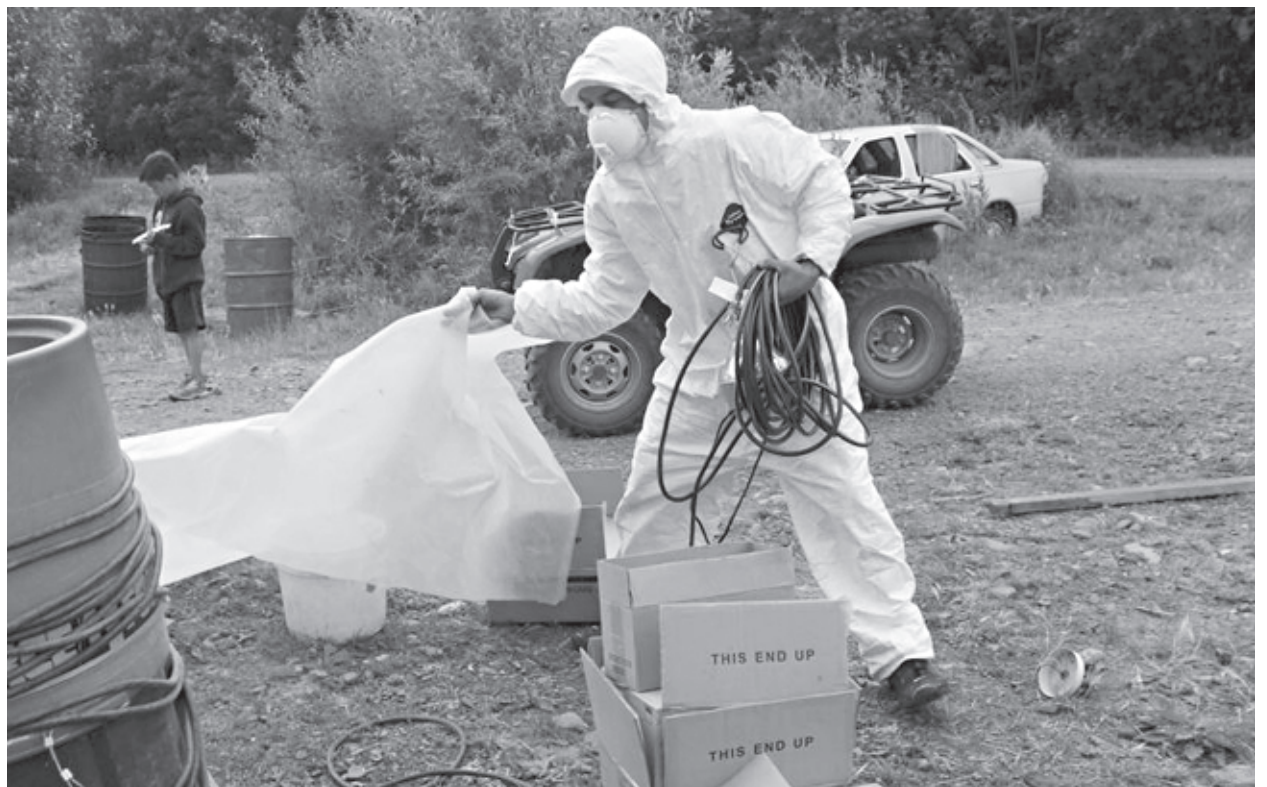
In Rampart, a weatherization crew member prepares to apply spray cellulose in the attic of a village home. In order to minimize contact with the material, workers "suit up", use breathing masks and follow other safety guidelines.
