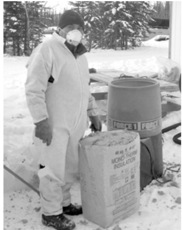
A weatherization employee prepares to add new insulation to the drum that feeds it into the adjacent dwelling in Tok. The project is aimed at cutting energy costs in the region's small communities.
